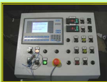
Electronic control by PLC
